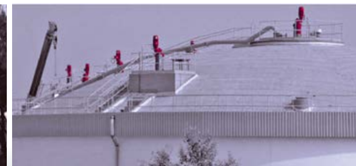
digestion tank (with several agitators) -- Algeria Baraki
