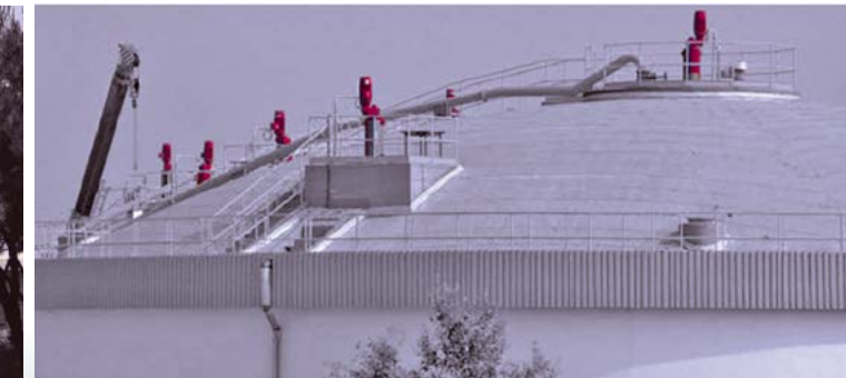
digestion tank (with several agitators) - - Algeria Baraki
